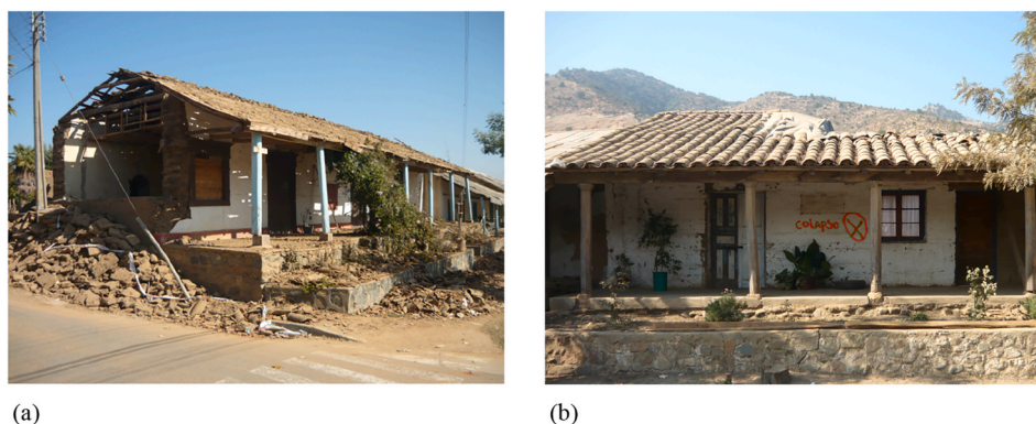
Fig. 3. (a) Traditional adobe buildings in Lolol damaged after the 2010 Mw 8.8 Maule earthquake in Chile. (b) Building misclassified as “Collapsed” and designated for demolition following field assessment.
